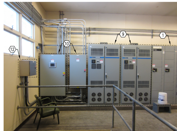
2 SCADA PANELS AND VFDs PHOTO E1.0 SCALE: NTS
