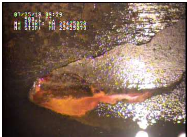
Photo 6-7 Missing Mortar w/ Minor Corrosion on 20" Force Main (~590' N of MH78)
