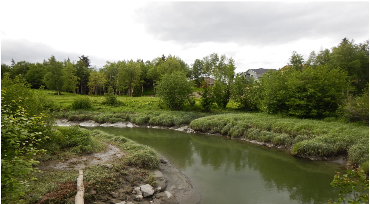
Figure 2: View of the bank stabilization area, looking upstream from the existing culverts and embankment.
