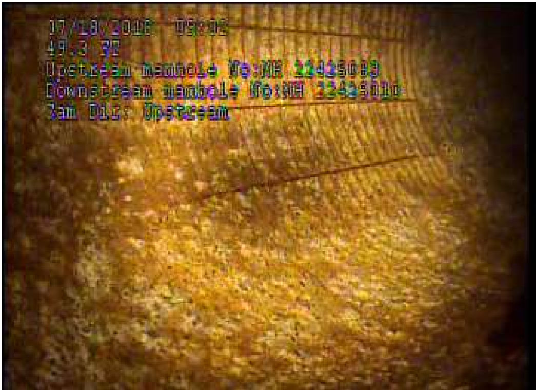
Photo 6-1 Exposed Rebar on Crown of 48" RCP
