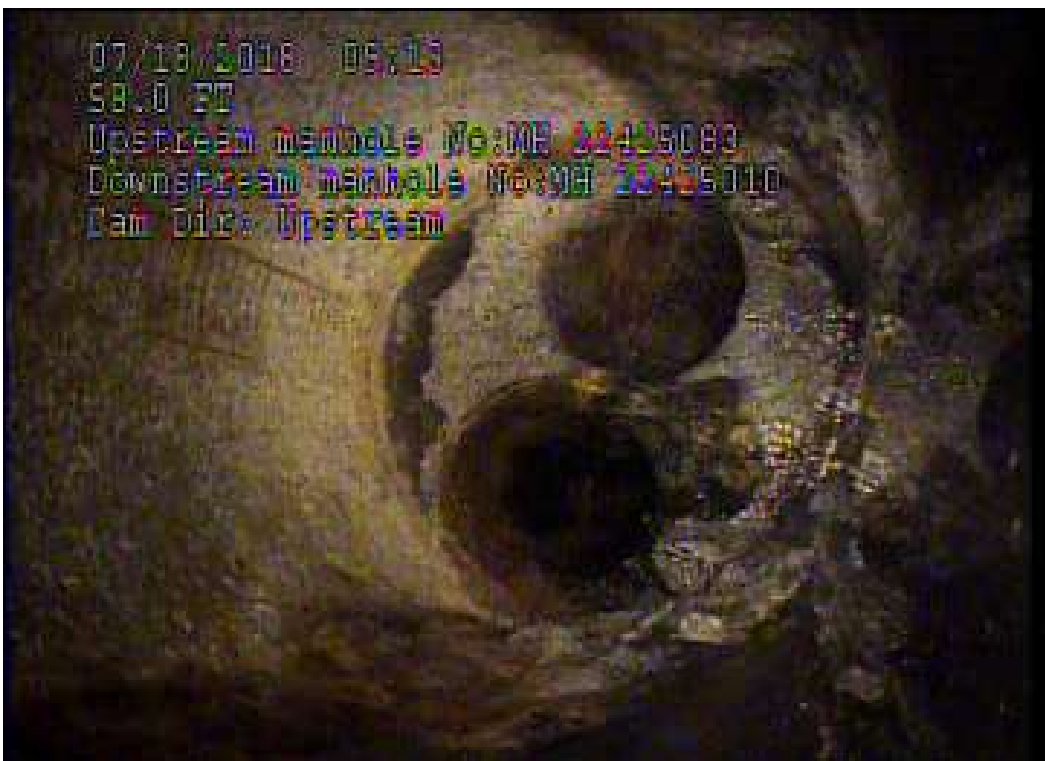
Photo 6-2 Gravity Junction w/ Exposed Rebar and Projecting Aggregate
