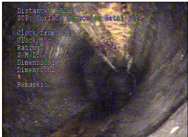
Photo 6-5 Corrosion on the Crown of 20" Force Main (beginning ~15' S of 45° bends)
