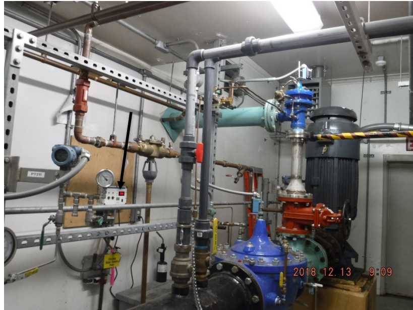
Photo 12-3: Existing PRVs and Chemical Analyzer
