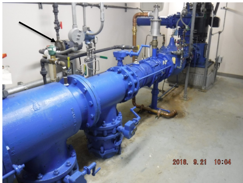
Photo 10-2: Existing Piping and Chemical feed Pump
