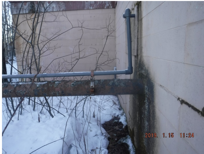
Photo 4-5: 6" CIP Discharge Line and 1-1/4" PVC Cooling line (North Side of Well House)
