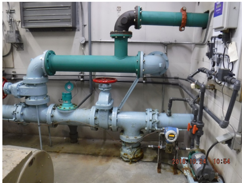
Photo 29-4: Existing Chemical Feed Pump and Skid
