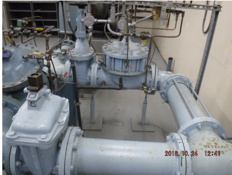
Photo 13-3: Existing Blow-Off PRV
