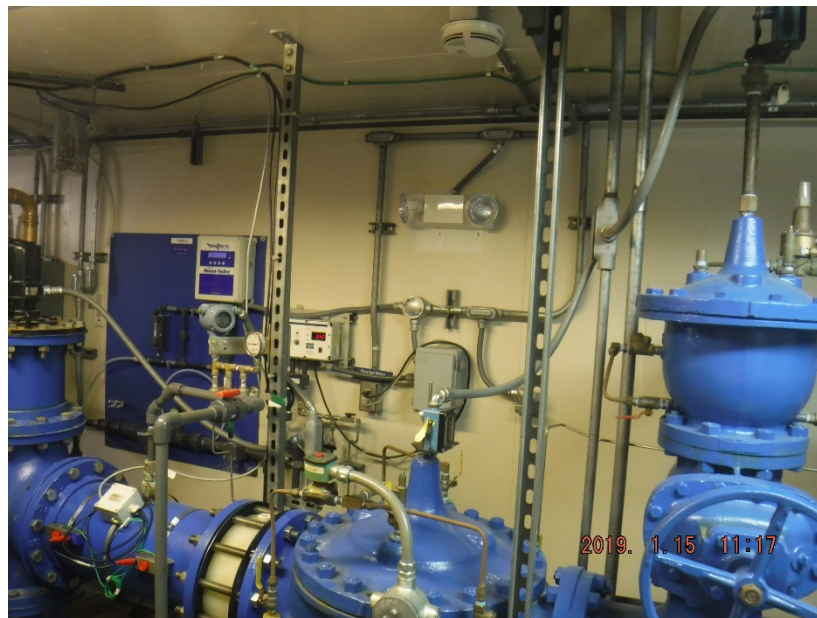
Photo 11-4: Existing Chemical Analyzer and Skid
