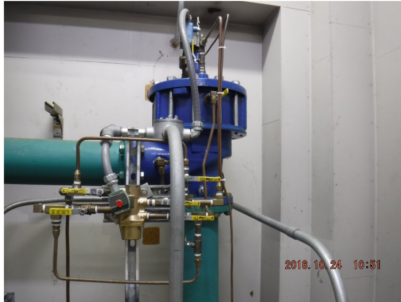
Photo 29-3: Existing Blow-Off PRV
