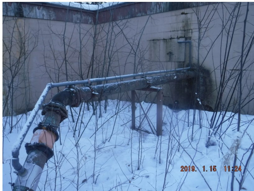
Photo 4-6: 6" CIP Discharge Line and 1-1/4" PVC Cooling line
