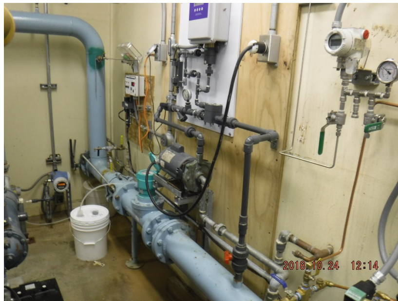
Photo 31-2: Existing Chemical Feed Pump and Chlorine Analyzer
