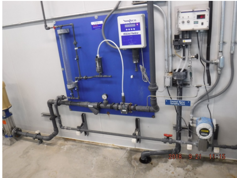
Photo 7-1: View of existing Chemical Analyzer system
