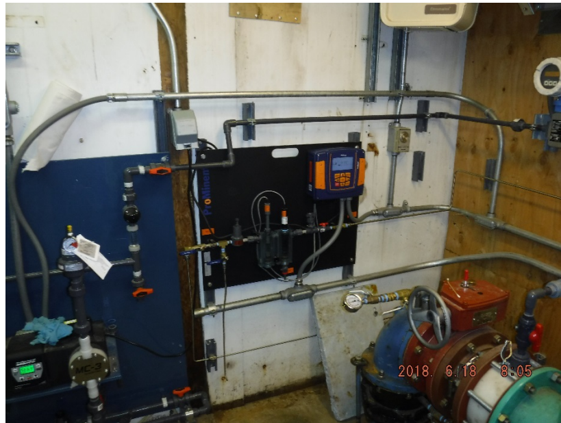
Photo 25-3: Existing Mixer, Chlorine Analyzer, Flow Meter, and Pump Skid
