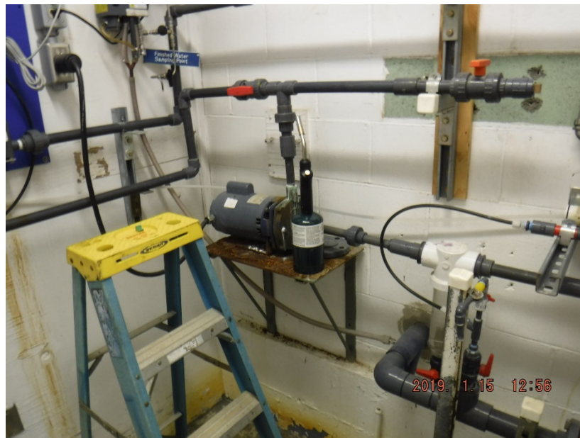
Photo 4-4: View of existing chemical feed pump
