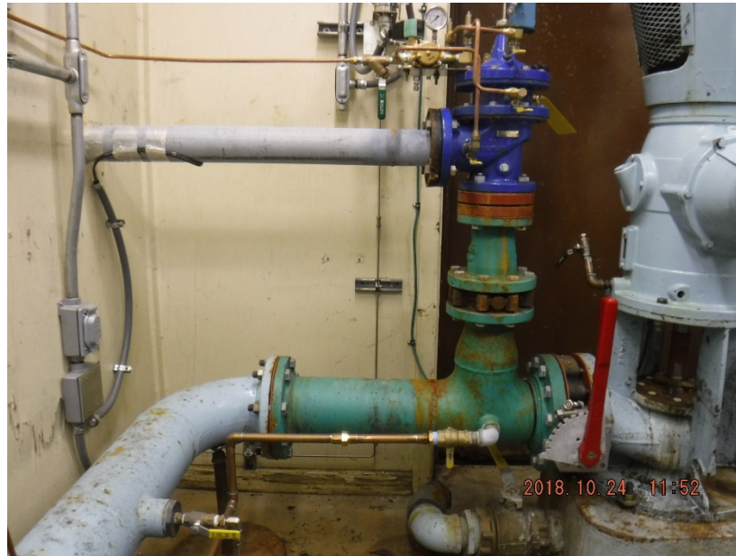
Photo 31-1: Existing Blow-Off PRV
