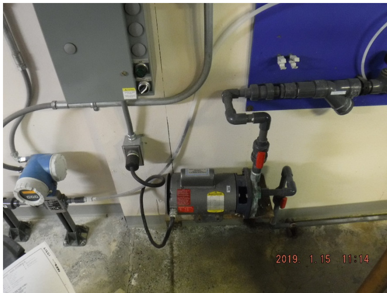
Photo 11-2: Existing Chemical Feed Pump
