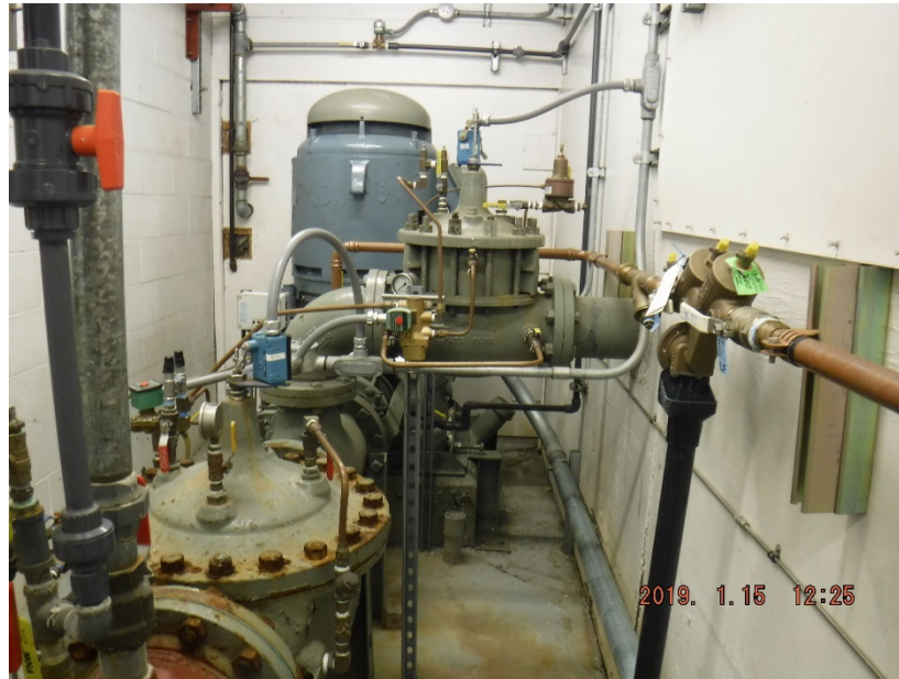
Photo 4-1: View of both existing PRVs from Generator Room
