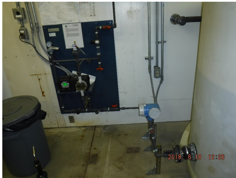
Photo 9-4: Existing Chemical Feed Pump and Skid
