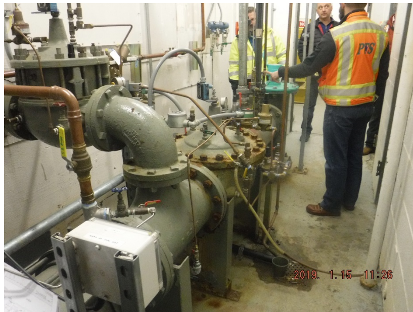
Photo 4-2: View of both existing PRVs from Well Head
