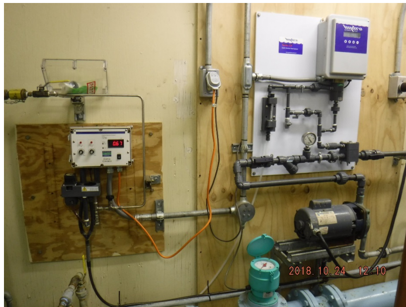
Photo 31-4: Existing Chemical Feed Pump, Skid, and Chlorine Analyzer.
