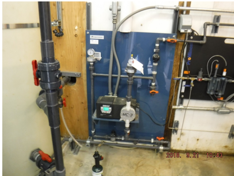
Photo 25-1: Existing Chemical Feed Pump and Skid
