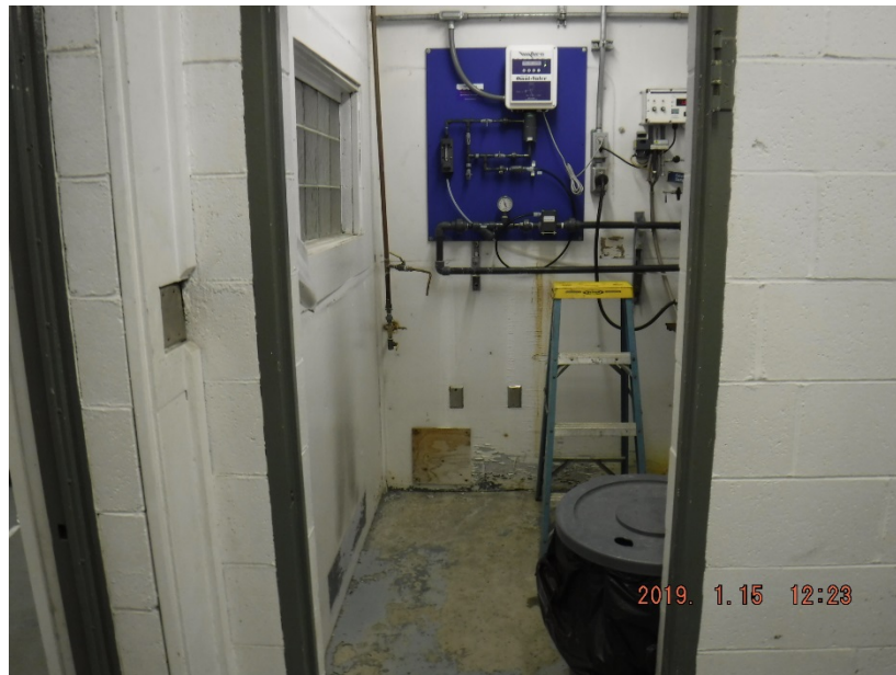
Photo 4-3: View of Chlorine Analyzer room from Well Room
