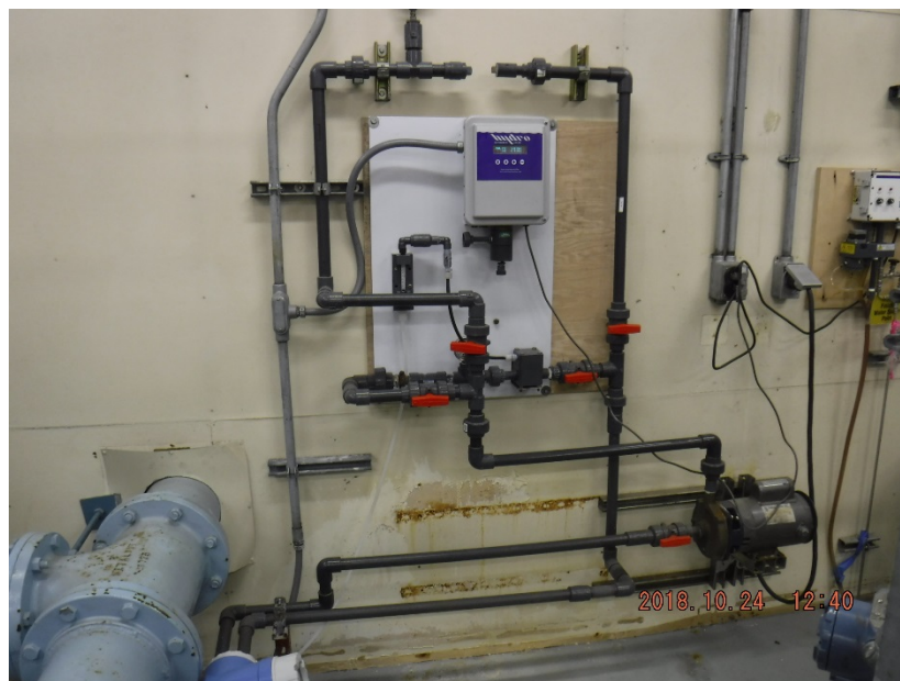
Photo 13-2: Existing Chemical Feed Pump and Skid
