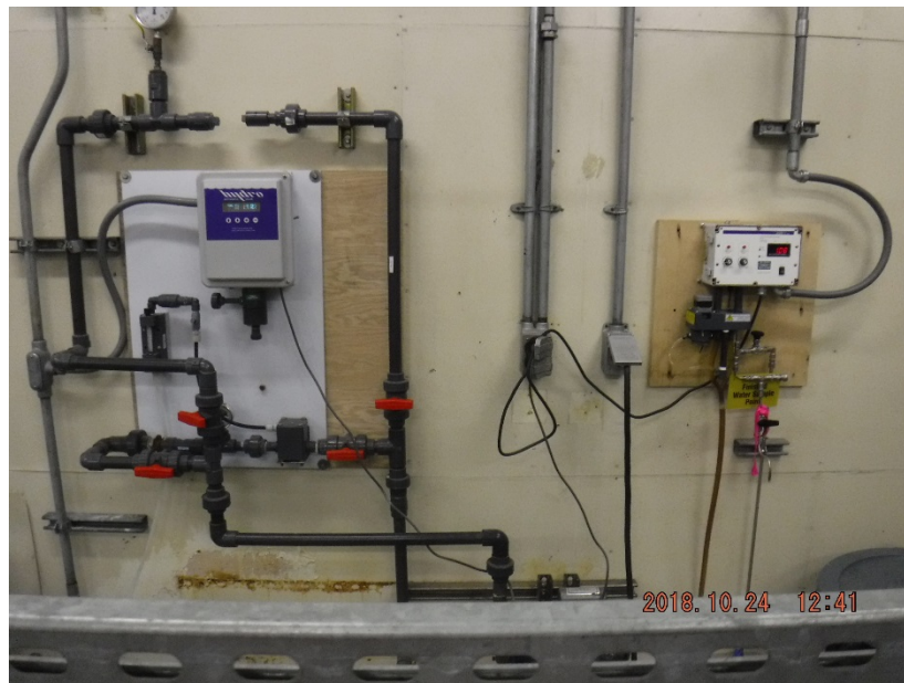
Photo 13-4: Existing Skid and Chemical Analyzer
