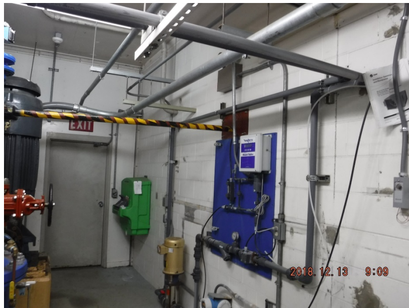
Photo 12-4: Existing Chemical Feed Pump and Skid
