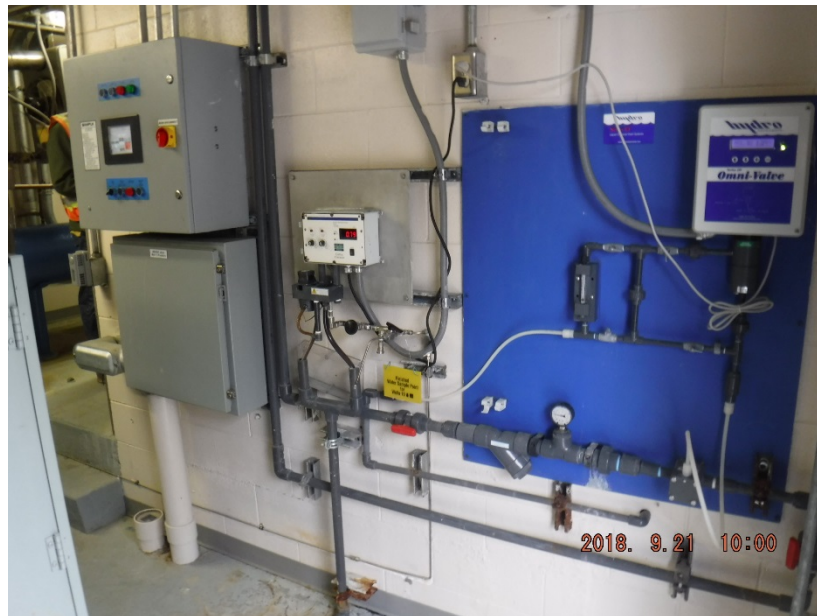
Photo 10-1: Existing Chemical Analyzer and Chemical Feed Skid
