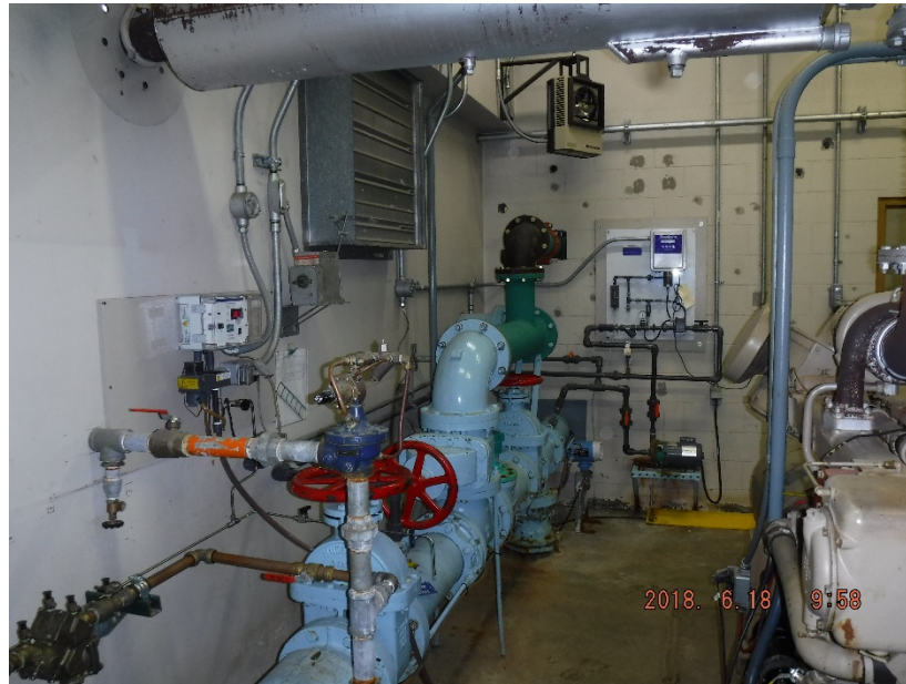
Photo 29-1: Existing Piping, Chemical Analyzer, and Chemical Feed Pump and Skid
