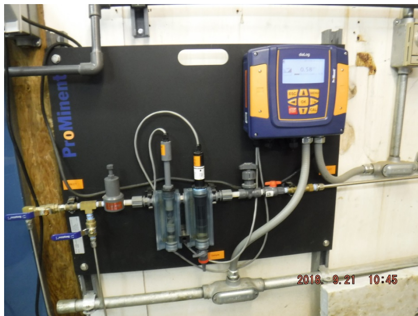
Photo 25-2: Existing Chlorine Analyzer
