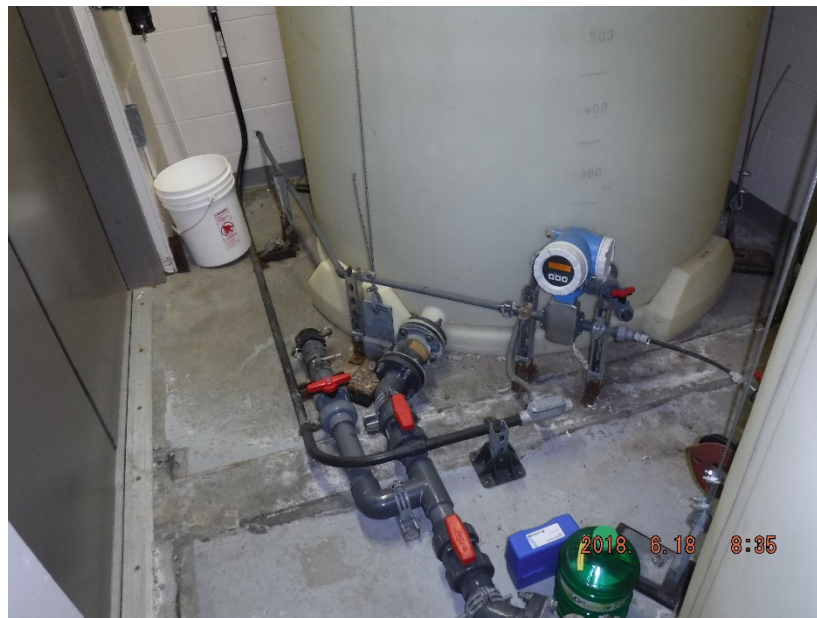
Photo 10-4: Chemical Storage Room that shares wall with Chemical Analyzer
