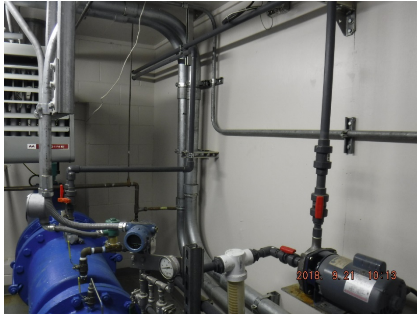
Photo 10-3: Existing Chemical Feed pump
