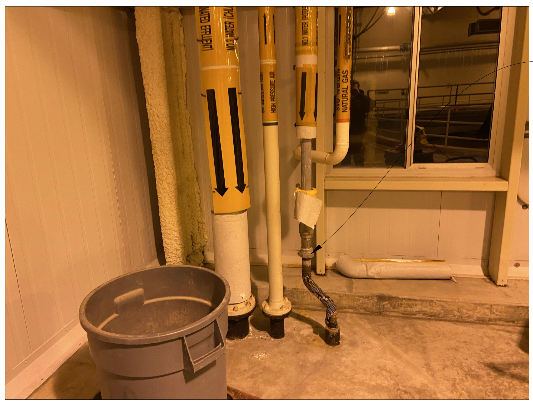
DAMAGED / MISSING W1 INSULATION TO BE REPLACED
