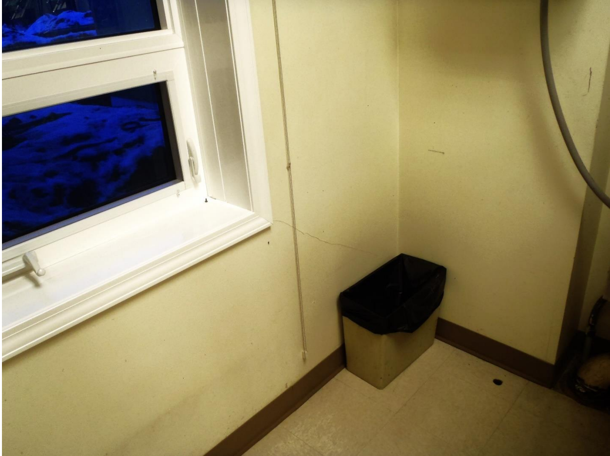
Drywall crack at window in Lab Area
