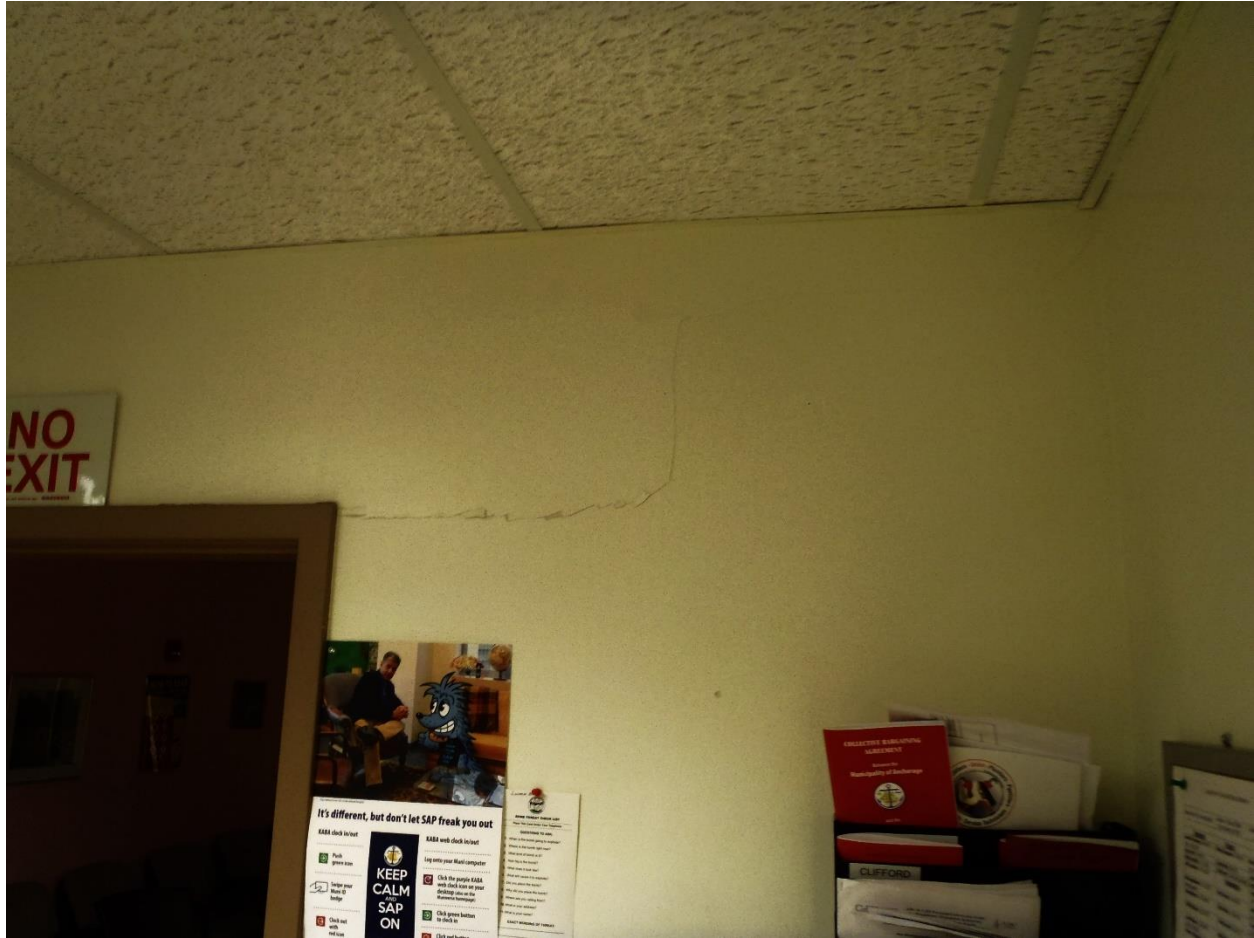
Drywall crack at doorway in Building 1 Break Room
