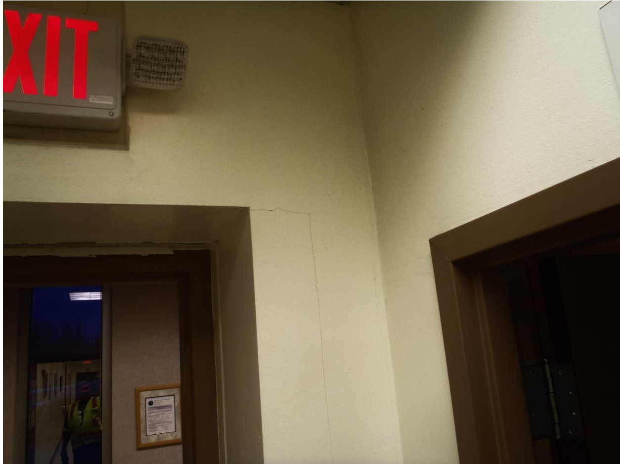
Drywall crack in Building 1 near Admin Area Vestibule Entry
