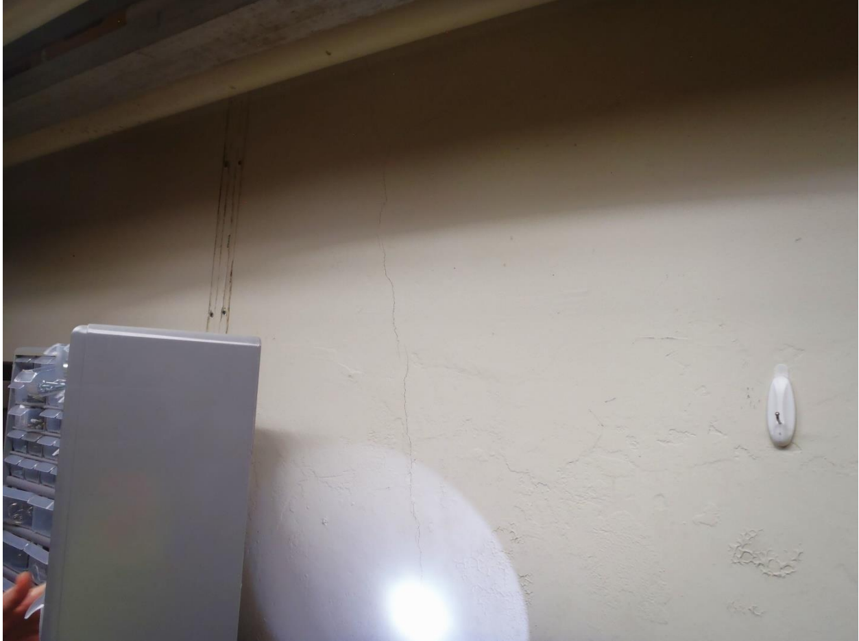
Drywall crack in Building 1 Shop Area
