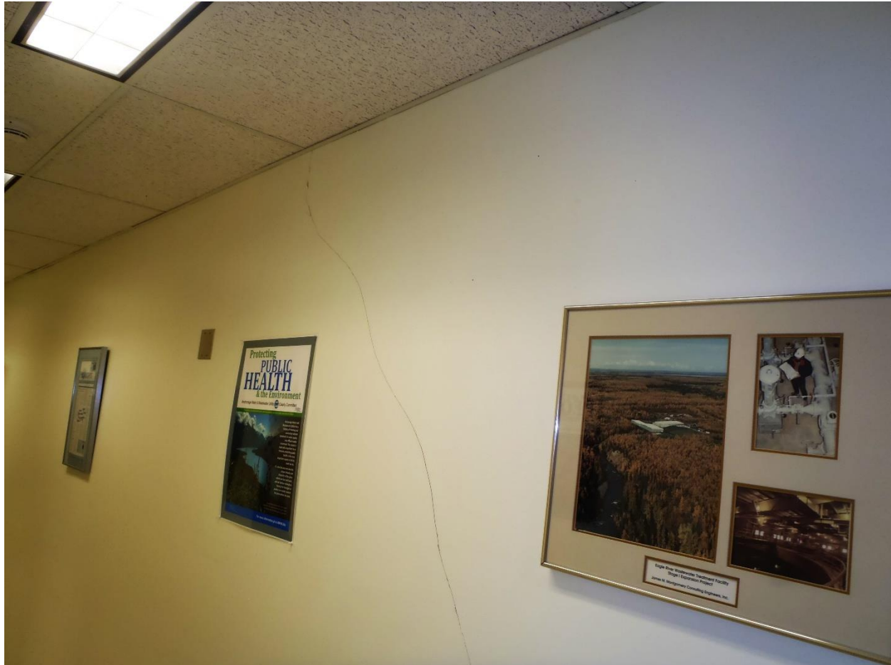
Drywall crack in Building 1 Admin Area Hallway
