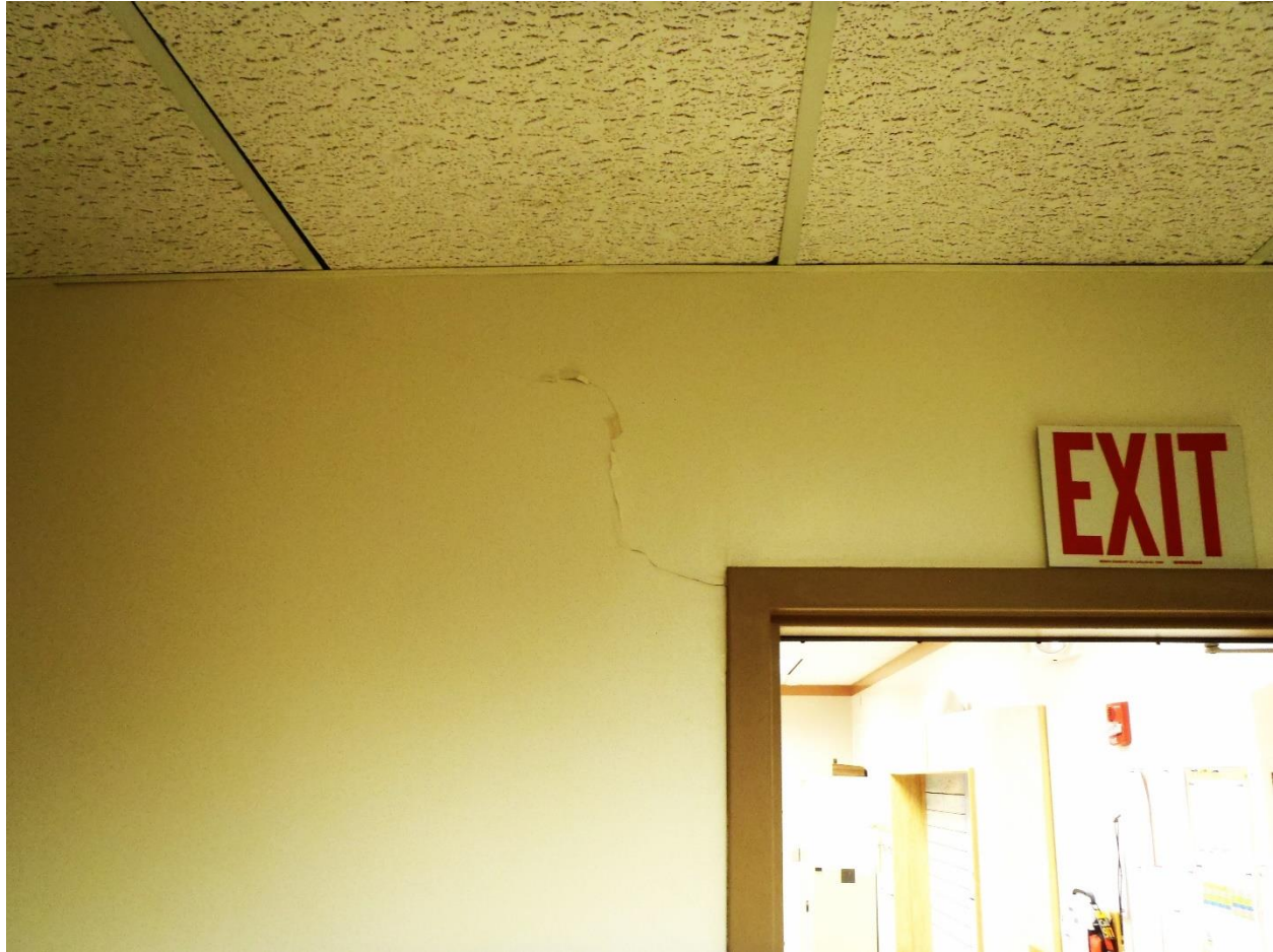
Drywall crack at doorway frame near Control Room in Building 1 Admin Area
