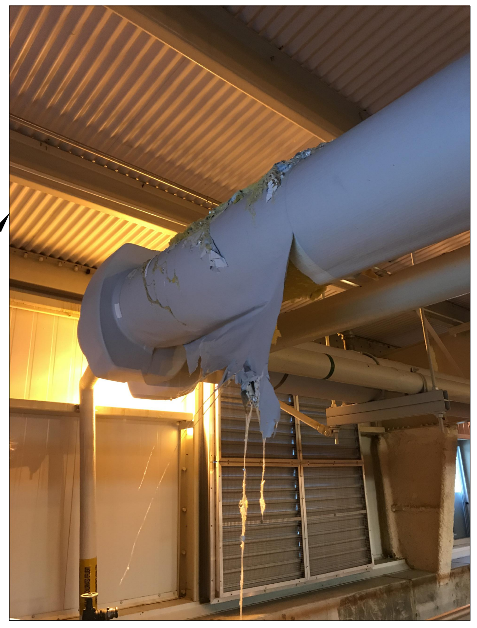
EXAMPLE OF W3 PIPING INSULATION DAMAGE TO BE REPAIRED IN THE AERATION BASIN BUILDING ALONG THE WEST WALL
