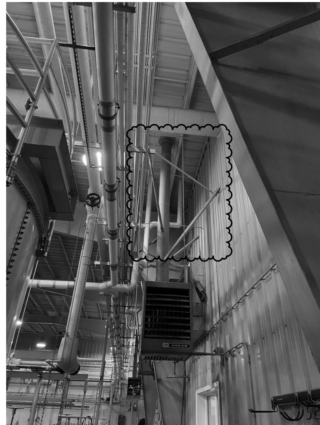
11 DAMAGED PIPE BRACING SCALE: NO SCALE
