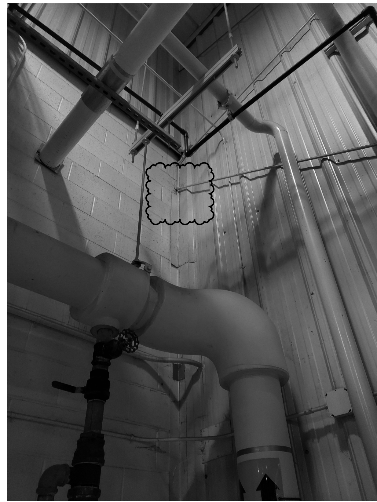
3 DAMAGED CMU WALL AT STEEL BRACE PENETRATION SCALE: NO SCALE
