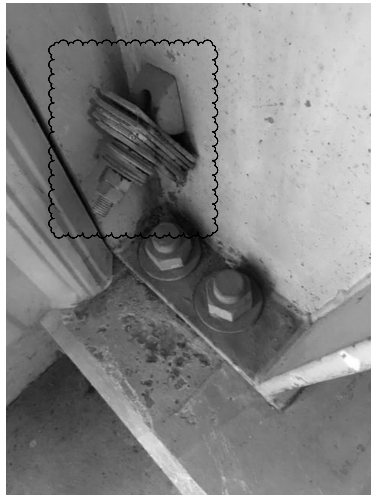
2 BUILT UP PLATE WASHERS DUE TO ELONGATED BRACES AT OCBF SCALE: NO SCALE
