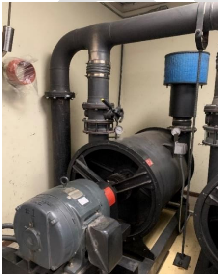
Photo 1 - Existing 75 Hp Spencer Turbo Compressor
