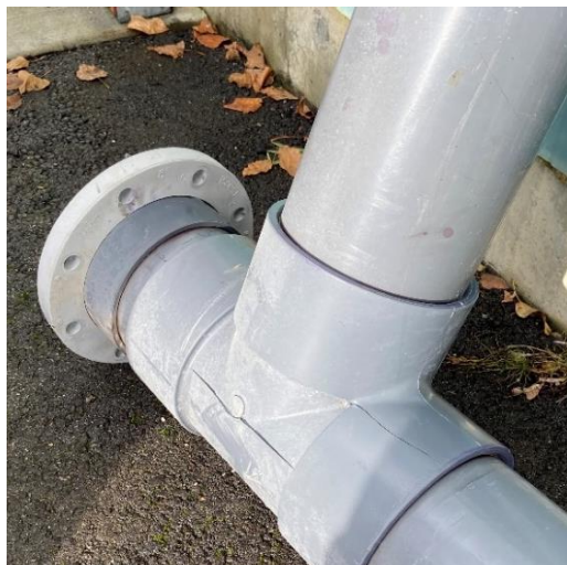
Photo 3 – Failure of Ex. 8-inch PVC Piping
