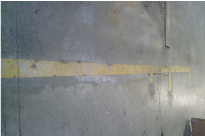
Photo 1: Reading # 21 – Floor Striping in Garage
