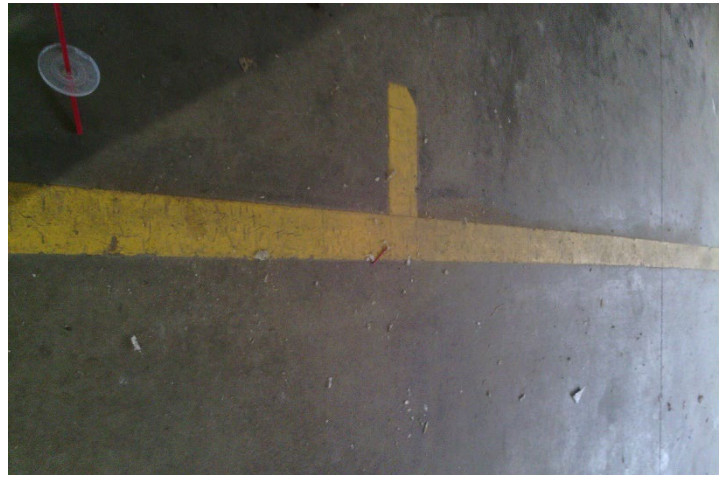
Photo 2: Reading # 22 – Floor Striping in Garage
