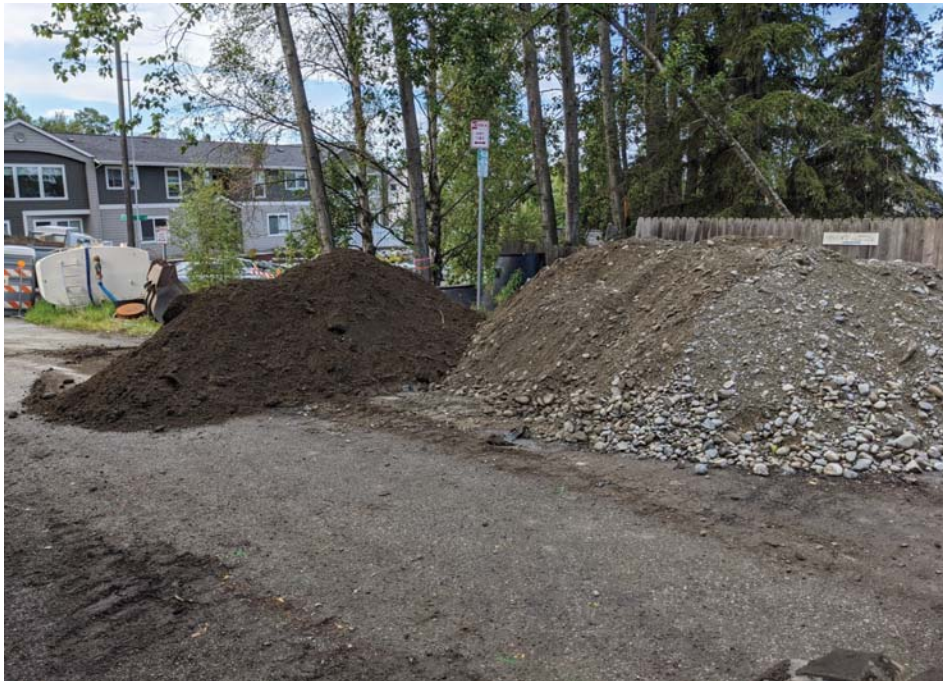
Photo 2: View looking west at the stockpiles of reusable material south of the excavation. In the background can be seen the dewatering storage tank on the corner of 6th Avenue and M Street.
