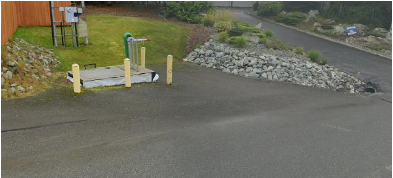
Knik View East PRV Vault 22499 Deer Park Dr.
