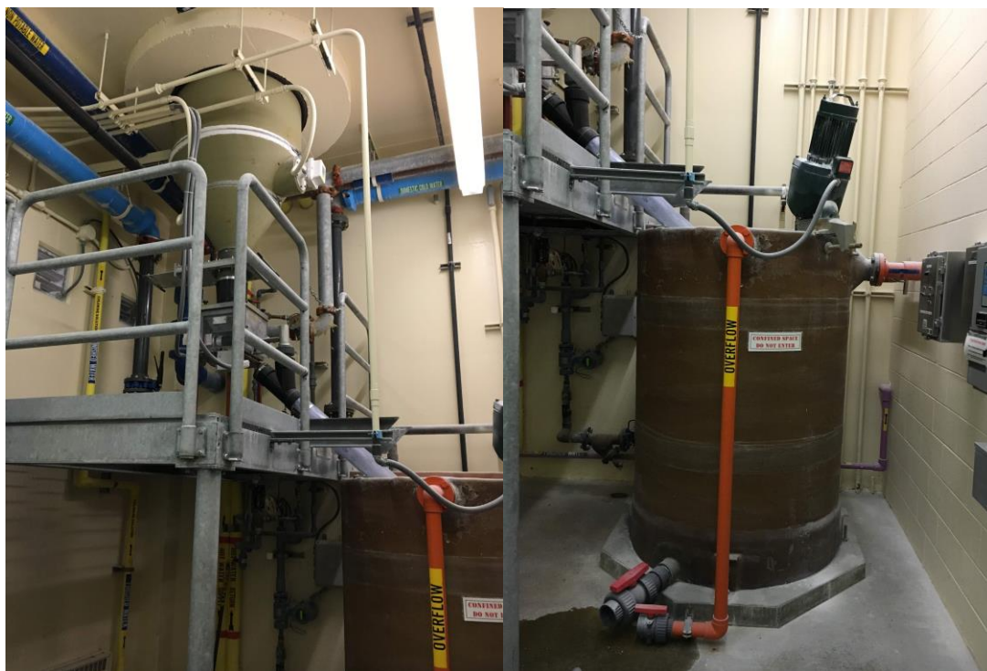
Figure 4-29 Existing Fluoride Storage Hopper, Dry Feeder and Mixing Tank
