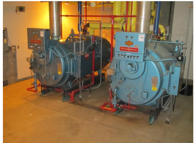
Figure 2-35 Boiler 4-HWB-1 and 4-HBW-2
