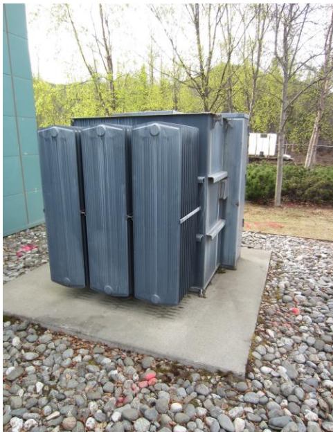
Figure 2-23 Medium Voltage Service Transformer
