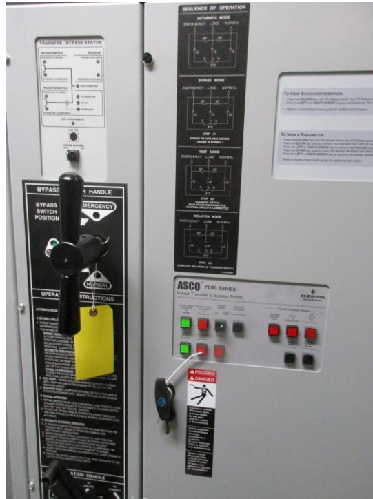
Figure 2-26 New Automatic Transfer Switch
