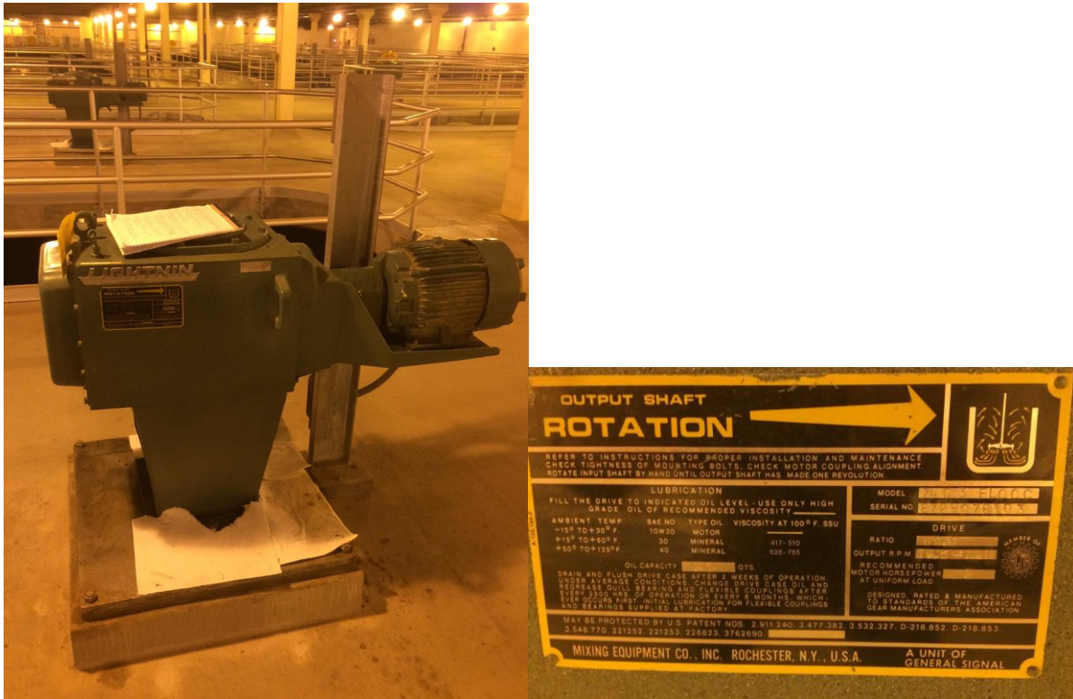
Figure 4-7 Existing Flocculator and Name Plate Data
