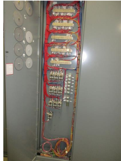
Figure 2-28 SCADA Interface Cabinet
