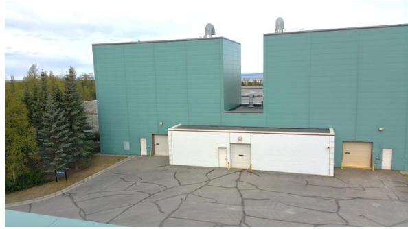
Figure 2-13 Cracked Pavement over Utilidor
