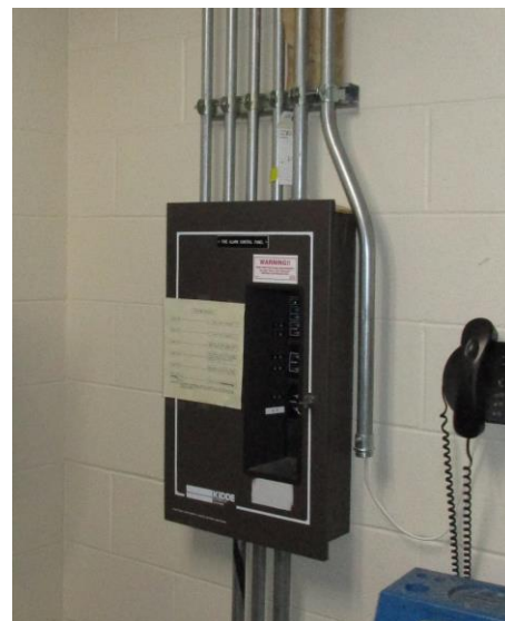
Figure 2-31 Fire Alarm Control Panel
