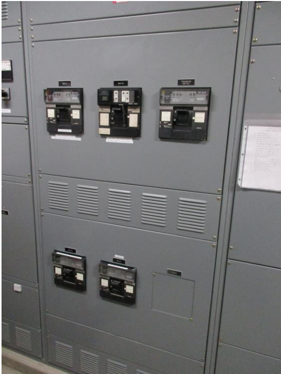
Figure 2-25 480 Volt Main Switchboard 'SDB'
