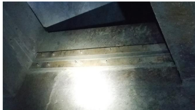
Figure 2-15b Leaking joint near riser box/floc basin transition
