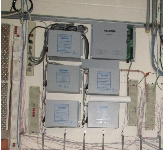
Figure 2-32 Public Address Head-End Equipment
