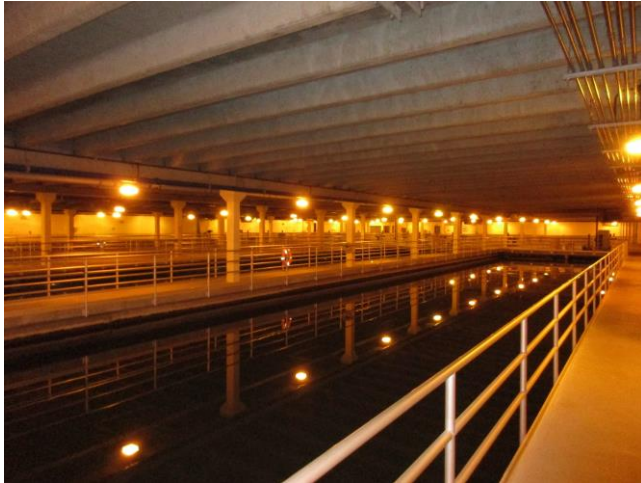
Figure 2-29 Floc and Sedimentation Basins
