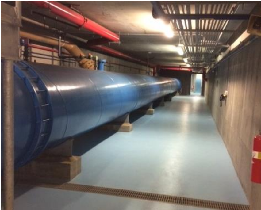
Figure 3-1 Existing Raw Water Pipe from the Energy Recovery Station
