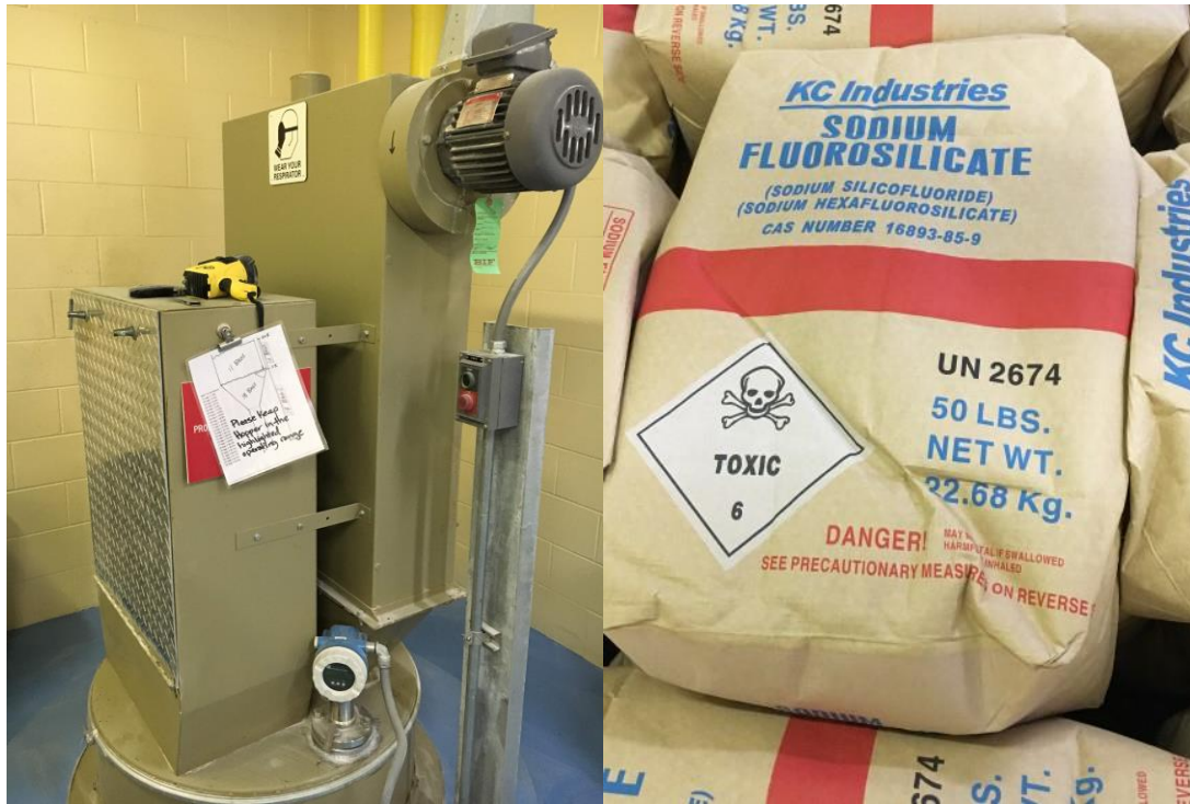
Figure 4-28 Existing Fluoride Bag Feeder and Bags of Sodium Fluorosilicate
