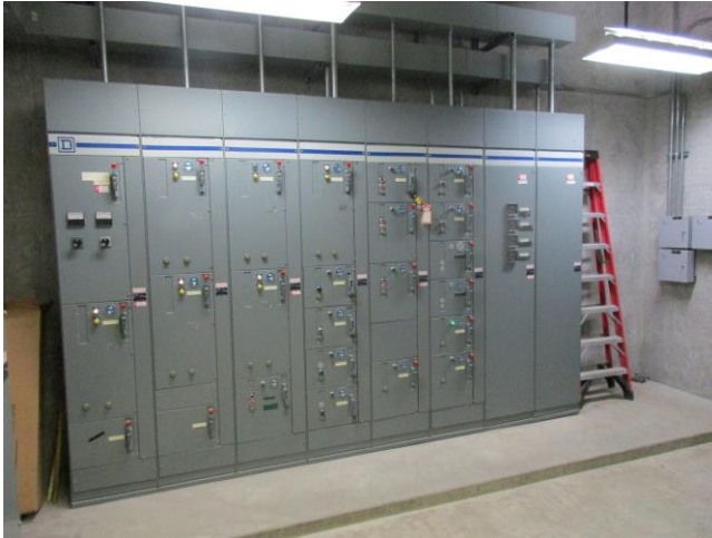
Figure 2-27 MCC-E Motor Control Center
