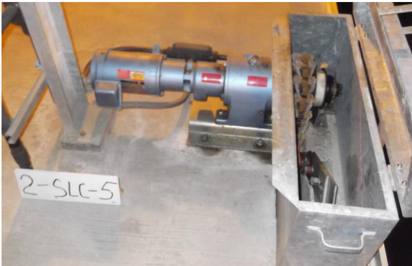
Figure 4-11 Existing Chain Drive Motor
