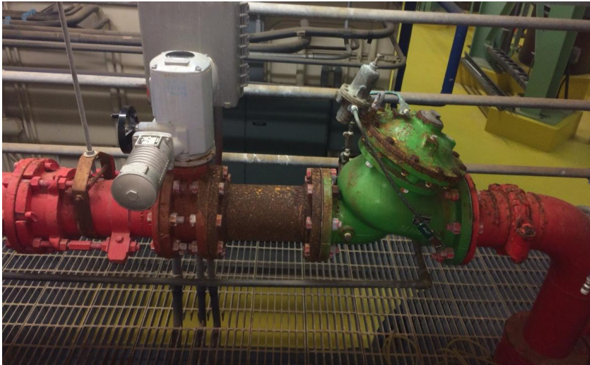
Figure 4-5 Flash mix feed water isolation valve and PRV
