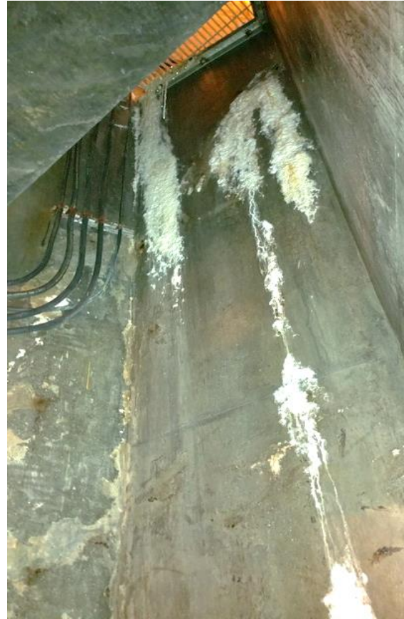
Figure 2-21 Calcium Weeping through Walls
