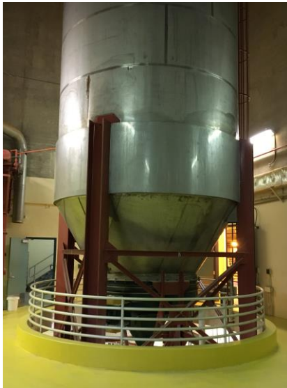
Figure 4-42 One of two ferric chloride silos with structural supports and floor opening.
