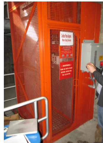
Figure 2-11 Intake Structure Elevator
