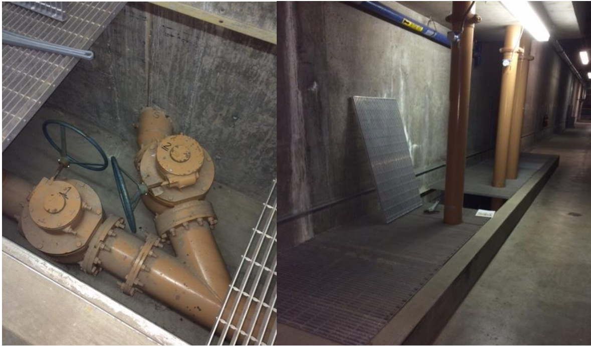
Figure 4-12 Two of three sedimentation drain valves
