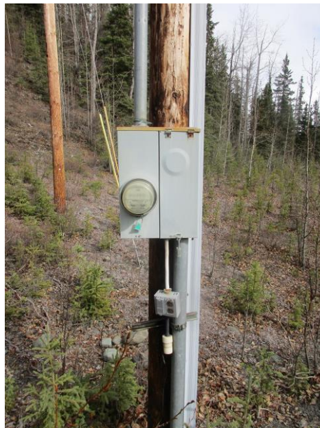
Figure 2-24 Portal Building Service Equipment
