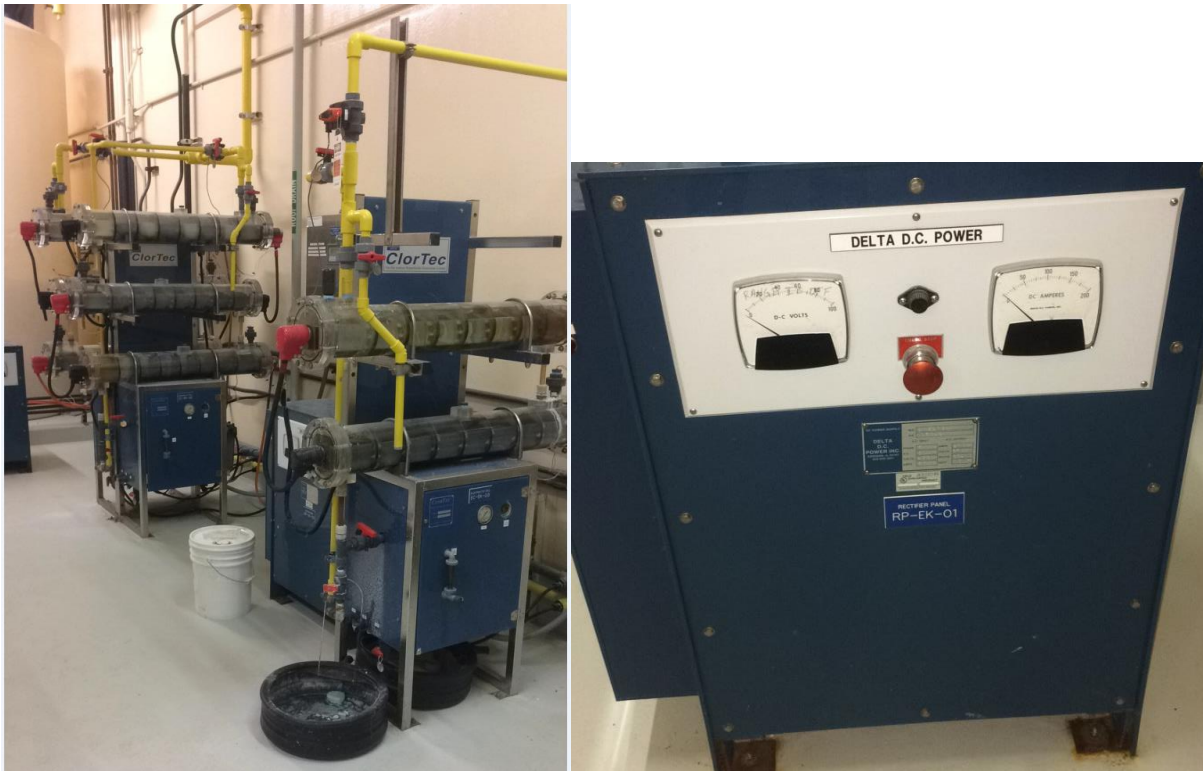
Figure 4-35 Existing ClorTec OSHG skids (left) and an OSHG system electrical rectifier (right)
