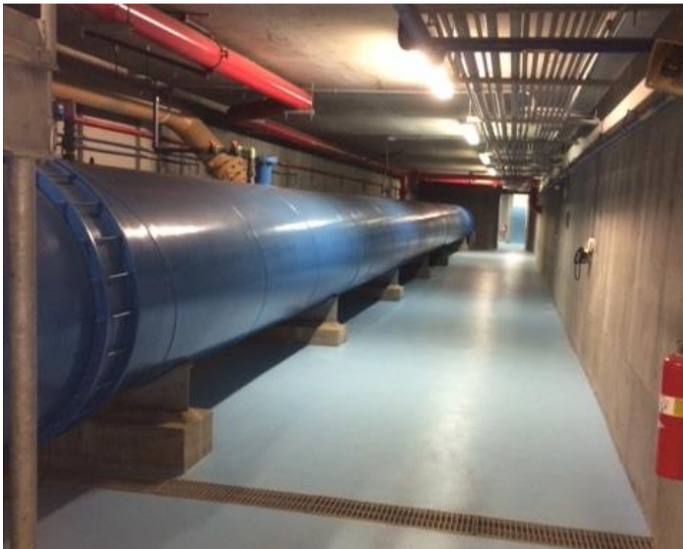
Figure 4-4 Existing Raw Water pipe from the Energy Recover Station also showing the mixing water and chemical injection on the top of the pipe.
