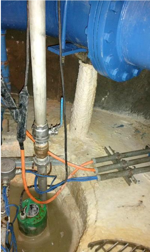
Figure 2-20 Calcium Build-up at Sump
