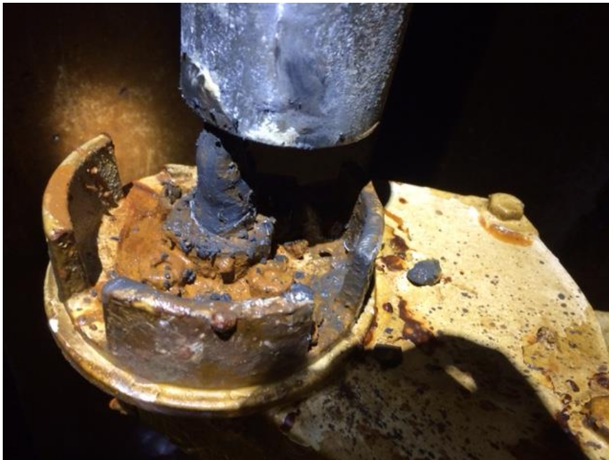
Figure 4-18 Clearwell drain valve corrosion and stem damage
