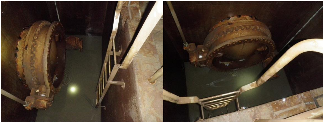
Figure 4-17 Clearwell influent (left) and effluent (right) valves and gear box/actuators
