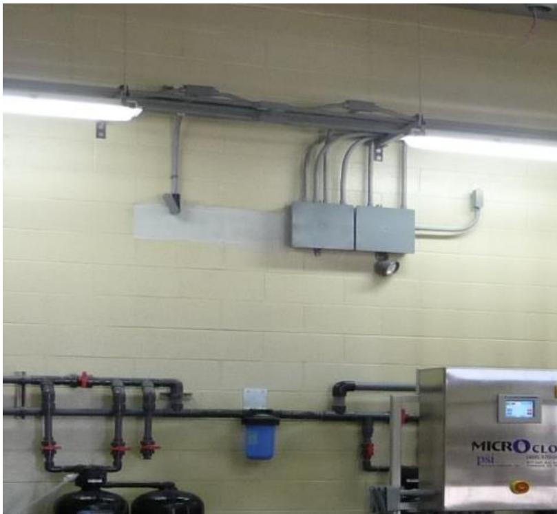
Figure 4-39 PSI MicroClor existing installed 2X200 ppd units [PSI]
