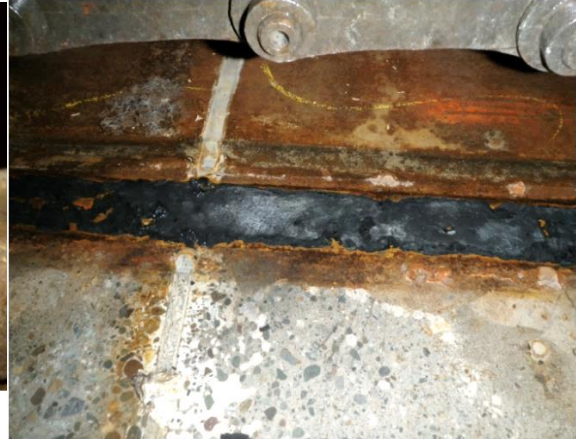
Figure 4-10 North Sediment Basin – Corroded Guide Shoe
