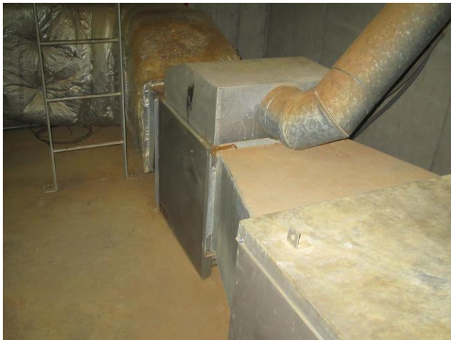
Figure 2-34 Duct heater 1-AHJ-1
