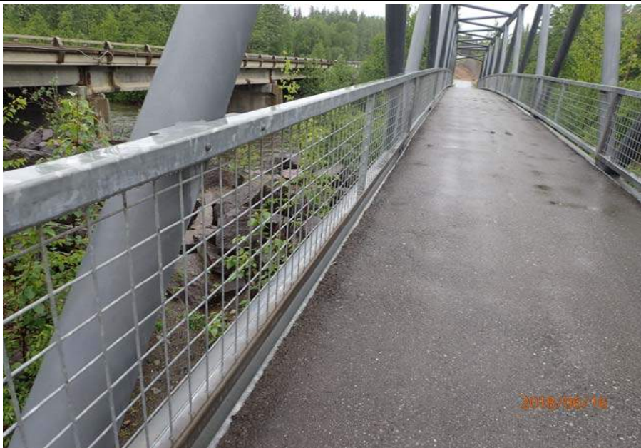
Bridge No. 6012 Br. Name Montana Cr Pedestrian Date 06/16/18 Inspector Sara Manning / Mary McRae Frame 15 Typical rail panel File P6160143.JPG
