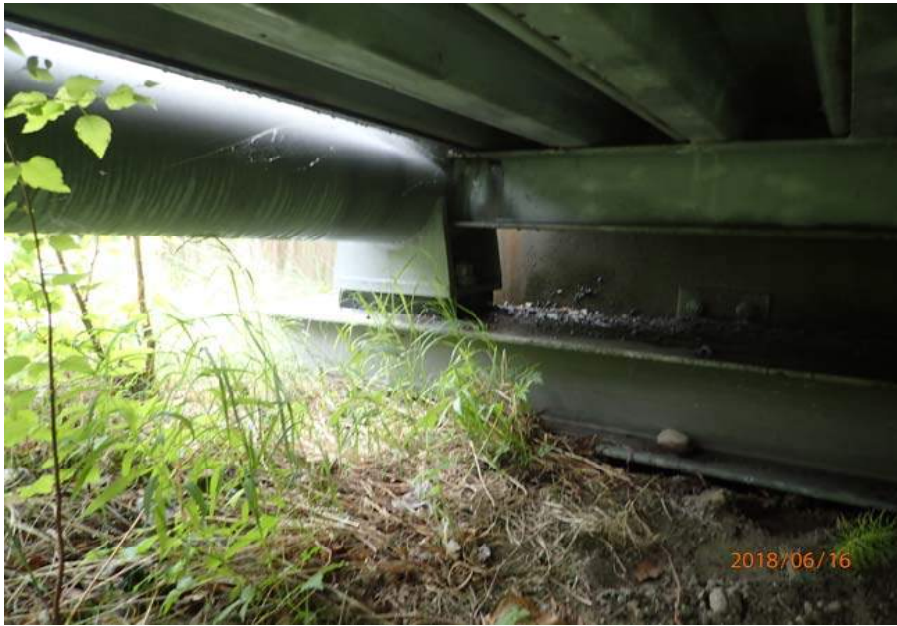
Bridge No. 6012 Br. Name Montana Cr Pedestrian Date 06/16/18 Inspector Sara Manning / Mary McRae Frame 17 Typical bearing (NE US shown) File P6160153.JPG
