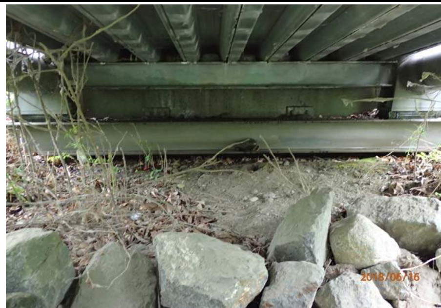
Bridge No. 6012 Br. Name Montana Cr Pedestrian Date 06/16/18 Inspector Sara Manning / Mary McRae Frame 8 FE abutment File P6160126.JPG
