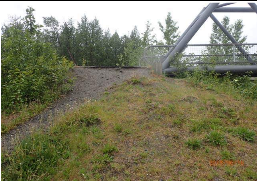
Bridge No. 6012 Br. Name Montana Cr Pedestrian Date 06/16/18 Inspector Sara Manning / Mary McRae Frame 19 Spalled asphalt, erosion gully NE US File P6160162.JPG
