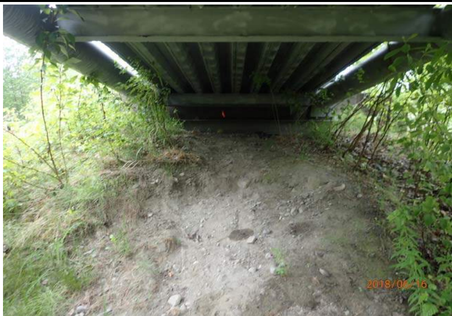
Bridge No. 6012 Br. Name Montana Cr Pedestrian Date 06/16/18 Inspector Sara Manning / Mary McRae Frame 7 NE abutment File P6160152.JPG
