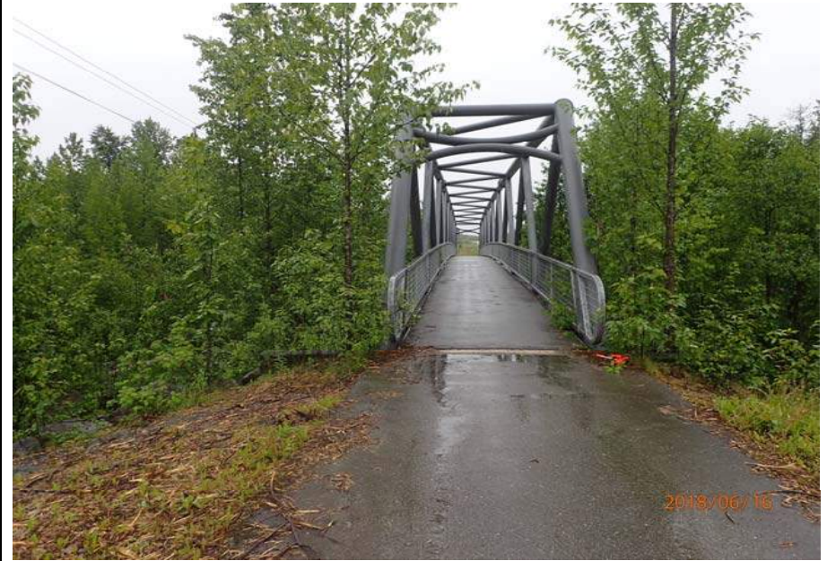
Bridge No. 6012 Br. Name Montana Cr Pedestrian Date 06/16/18 Inspector Sara Manning / Mary McRae Frame 2 Back at bridge File P6160123.JPG
