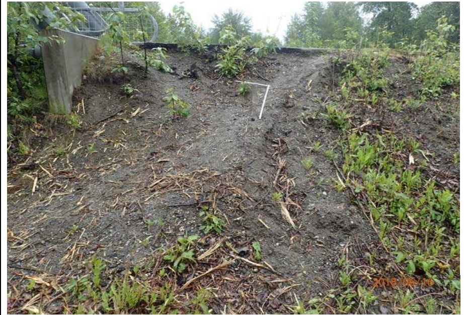
Bridge No. 6012 Br. Name Montana Cr Pedestrian Date 06/16/18 Inspector Sara Manning / Mary McRae Frame 18 Spalls, exposed geotextile, erosion NE DS File P6160146.JPG
