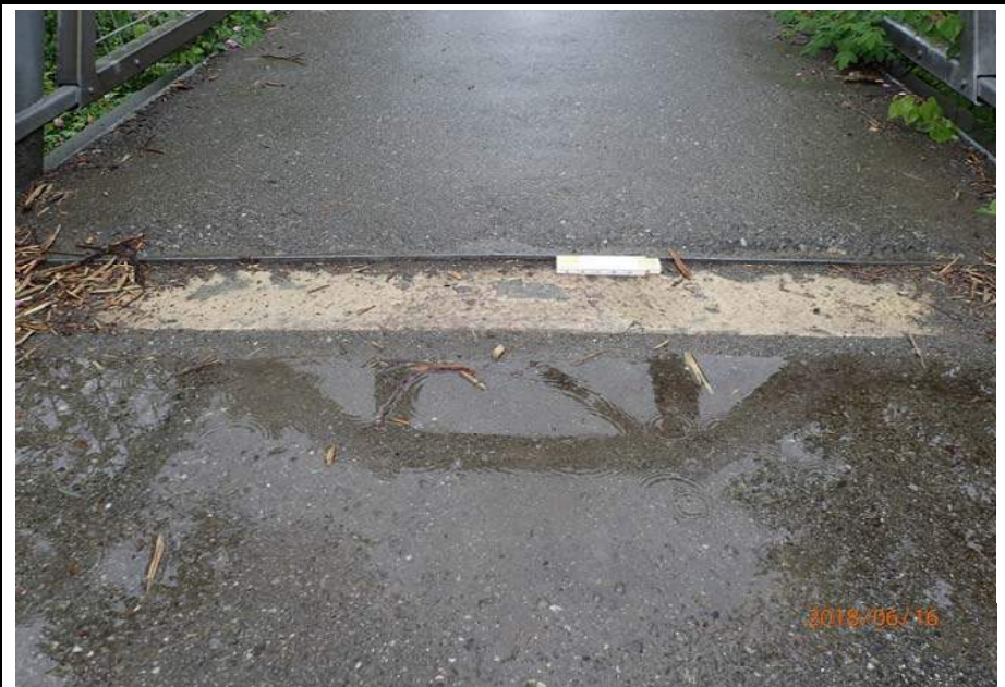
Bridge No. 6012 Br. Name Montana Cr Pedestrian Date 06/16/18 Inspector Sara Manning / Mary McRae Frame 20 Bump at FE joint File P6160136.JPG
