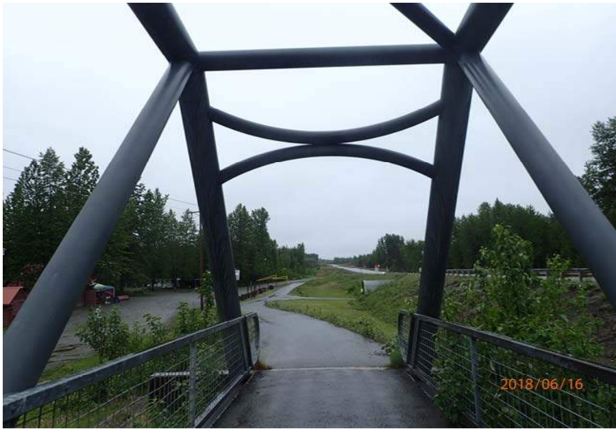
Bridge No. 6012 Br. Name Montana Cr Pedestrian Date 06/16/18 Inspector Sara Manning / Mary McRae Frame 9 NE portal File P6160144.JPG
