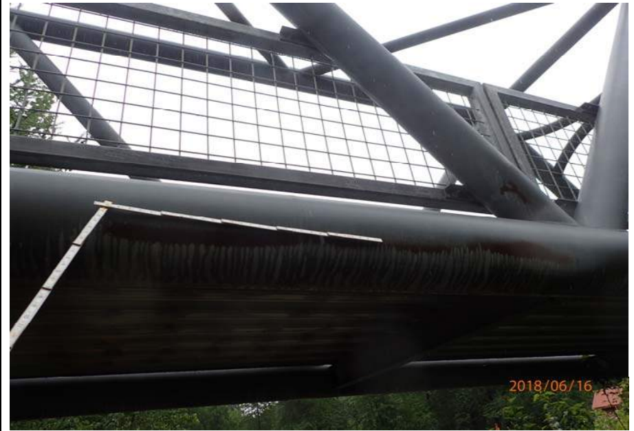
Bridge No. 6012 Br. Name Montana Cr Pedestrian Date 06/16/18 Inspector Sara Manning / Mary McRae Frame 14 Rust on bottom chord typical NE File P6160151.JPG
