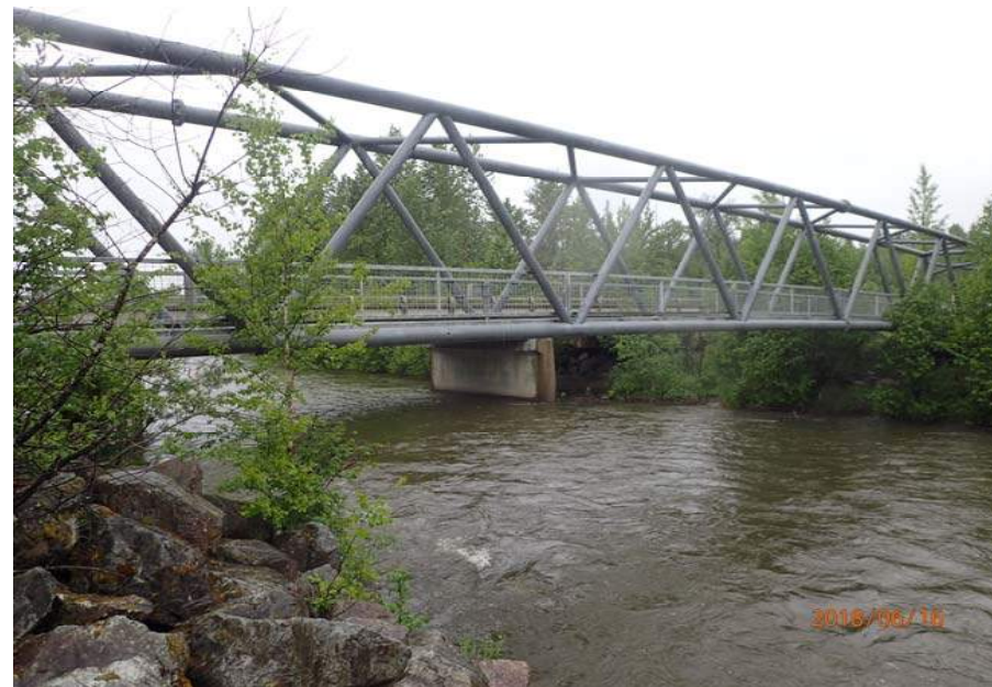
Bridge No. 6012 Br. Name Montana Cr Pedestrian Date 06/16/18 Inspector Sara Manning / Mary McRae Frame 6 US elevation File P6160160.JPG
