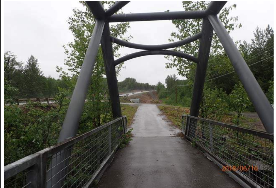
Bridge No. 6012 Br. Name Montana Cr Pedestrian Date 06/16/18 Inspector Sara Manning / Mary McRae Frame 10 FE portal File P6160137.JPG
