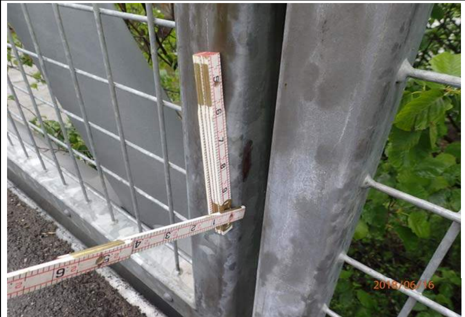
Bridge No. 6012 Br. Name Montana Cr Pedestrian Date 06/16/18 Inspector Sara Manning / Mary McRae Frame 16 Typical surface rust at rail panel ends File P6160139.JPG
