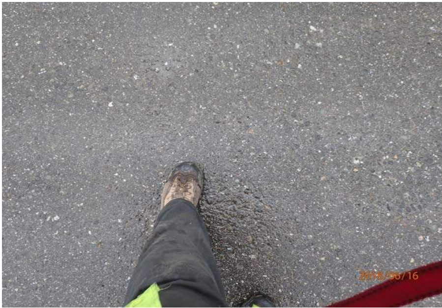
Bridge No. 6012 Br. Name Montana Cr Pedestrian Date 06/16/18 Inspector Sara Manning / Mary McRae Frame 13 Wearing surface File P6160142.JPG
