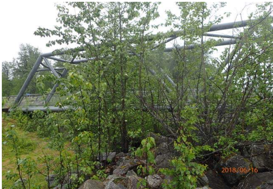
Bridge No. 6012 Br. Name Montana Cr Pedestrian Date 06/16/18 Inspector Sara Manning / Mary McRae Frame 5 US elevation File P6160161.JPG
