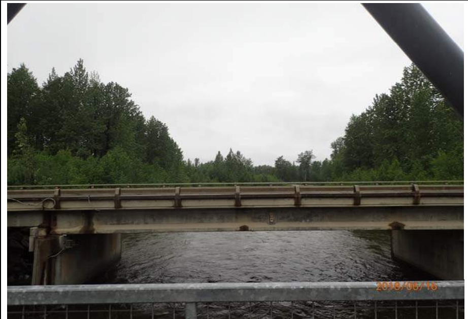
Bridge No. 6012 Br. Name Montana Cr Pedestrian Date 06/16/18 Inspector Sara Manning / Mary McRae Frame 4 Looking DS File P6160115.JPG
